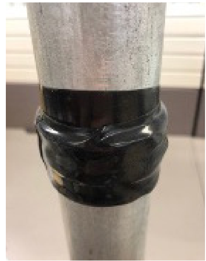
FIGURE 20: Tape Over Seal
